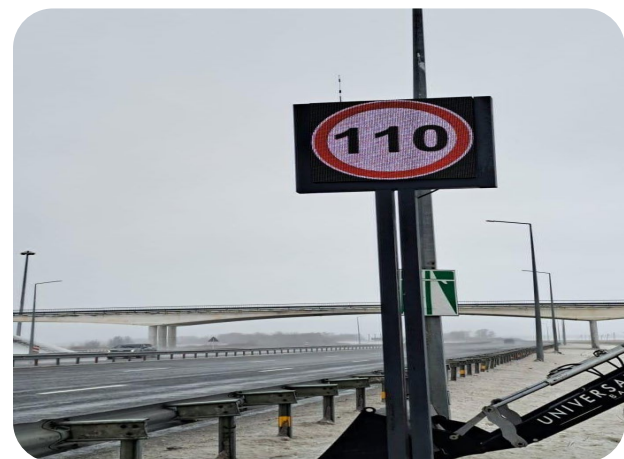
VARIABLE MESSAGE SIGNS (VMS)
